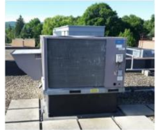
Rooftop Packaged Unit
