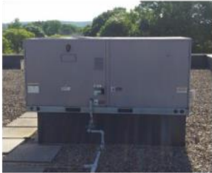
Rooftop Packaged Unit
