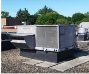
Rooftop Packaged Unit
